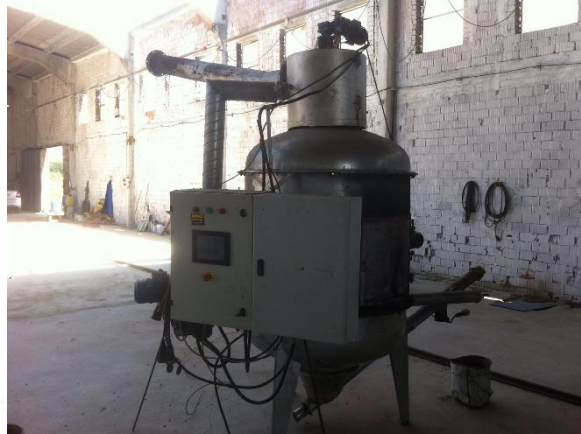
Figure 3. Turbulent combustion incinerator at working place.
