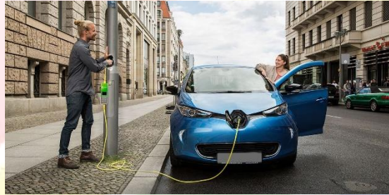
Fig.13. Charge Points From Electric Lighting Pole [16]
