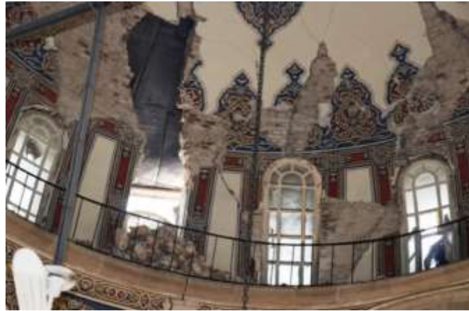
Figure 6. Damages of Malatya Hacı Yusuf Taş Mosque after earthquake (URL 7)
